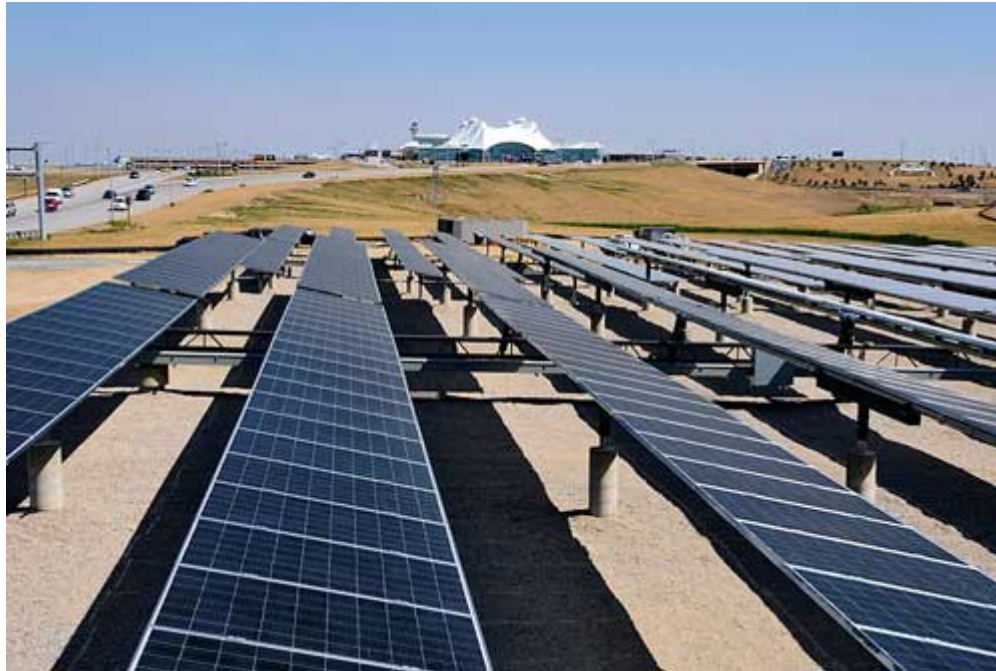
Denver International Airport is the fifth busiest airport in the U.S., serving nearly 50 million passengers annually; its solar system is one of the largest at any airport nationwide.
