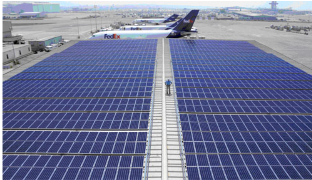
Sharp solar installations like this one at FedEx's distribution center help commercial enterprises reduce operating costs, increase efficiencies and develop strategies to achieve sustainability.
