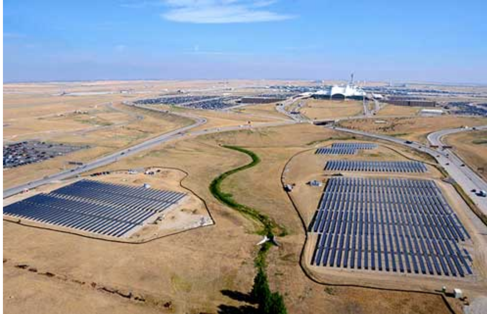
The highly visible Sharp solar system at the entrance to the Denver International Airport covers seven and a half acres, an area equivalent to seven football fields.
