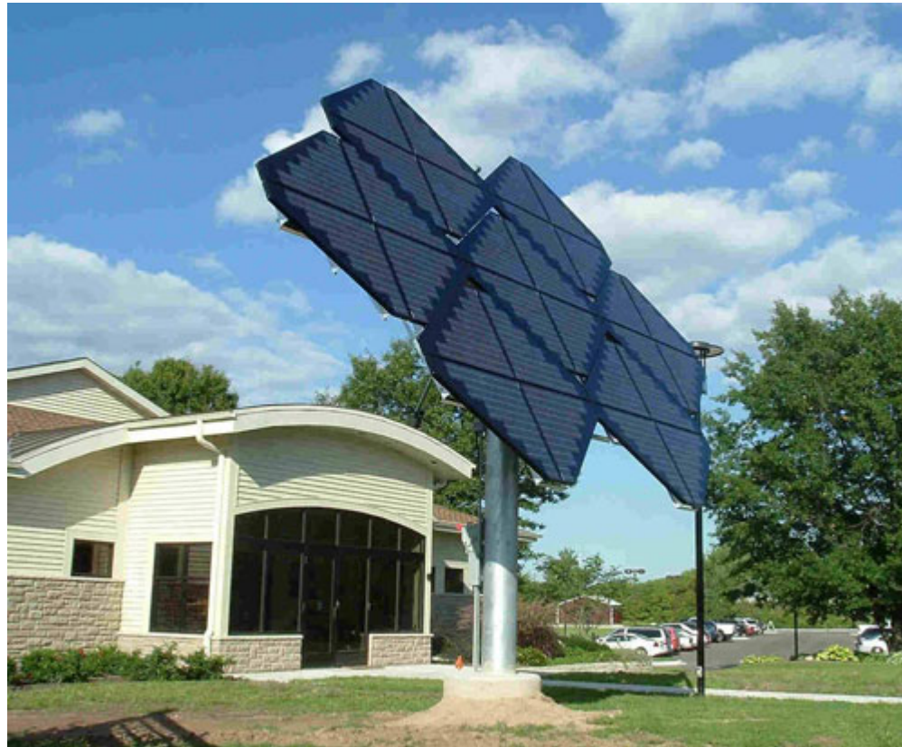
In this creative installation, Sharp's triangular modules are installed on a tracker that continually re-orientes them towards the sun, maximizing the amount of power they generate.
