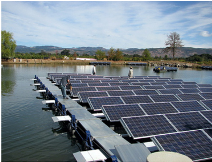
Almost 1000 Sharp solar panels were secured to pontoons to create an innovative "Floatovoltaic" solar array
